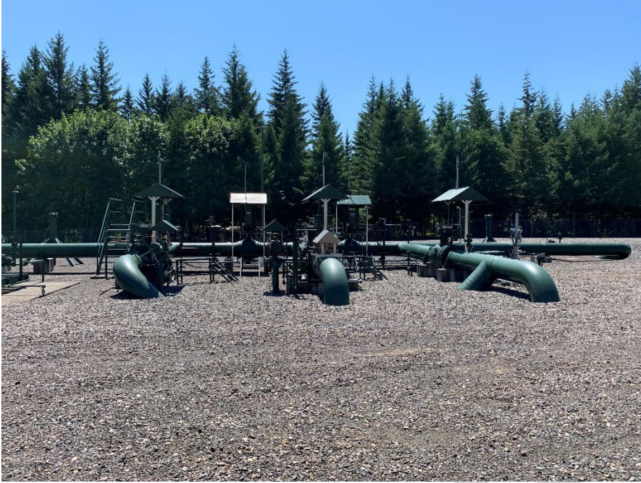
Looking south at inlet piping for three compressors at Willard station.
