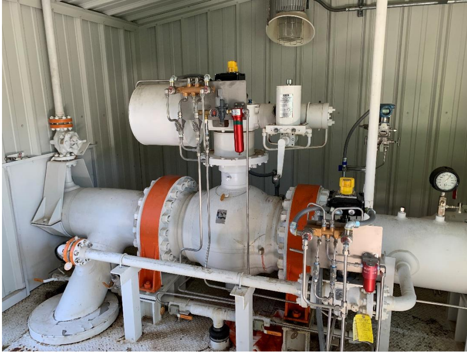
Unit 1 Suction valve. Note indicator is showing closed.
