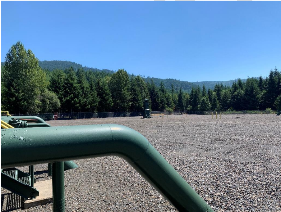
Looking east from outside Unit 1 suction valve building at vent stack. Pipe in foreground is 16" Unit 1 inlet.
