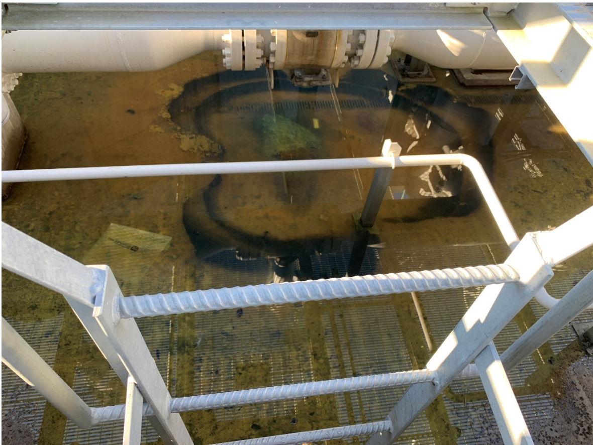
Photo 5 —looking north into containment area with leaked product.
