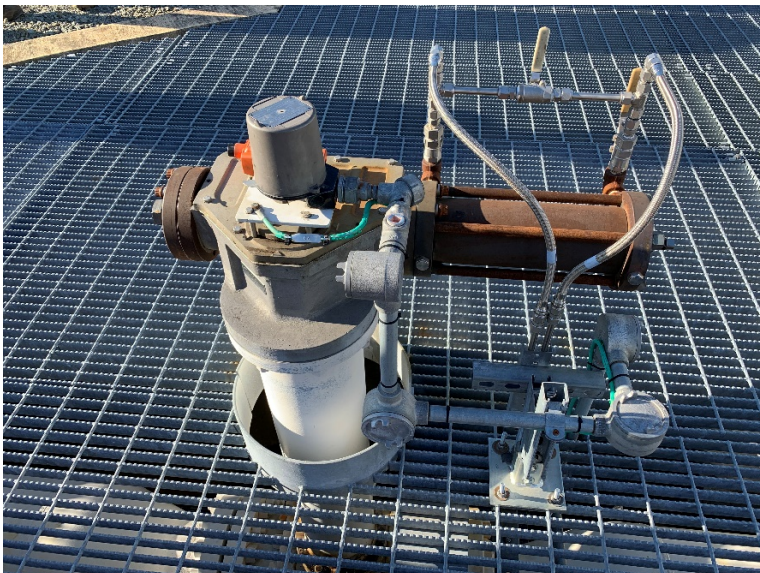
Photo 3 —looking north at Valve actuator and grating over containment area.
