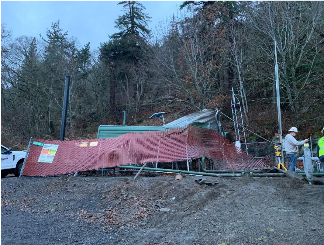
Figure 3: Photo taken at Hood River Meter Station on December 21, 2021 showing damage from the vehicle collision.
