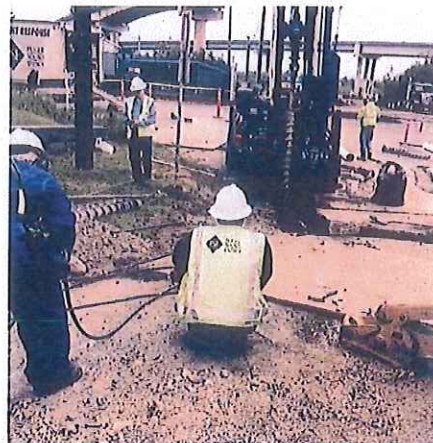
Figure 5. Remote control movement of drill away from damaged gas line and PSE fire watch.
