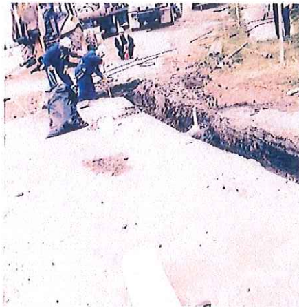
Figure 6. Exposure and assessment of damaged gas line and PSE fire watch.
