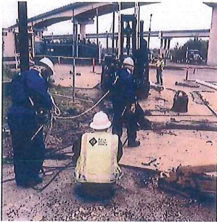
Figure 4. Remote control movement of drill away from damaged gas line and PSE fire watch.
