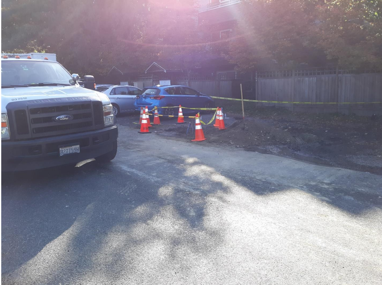
5-Photo of extra excavation used to squeeze off the flow of gas from the North.
