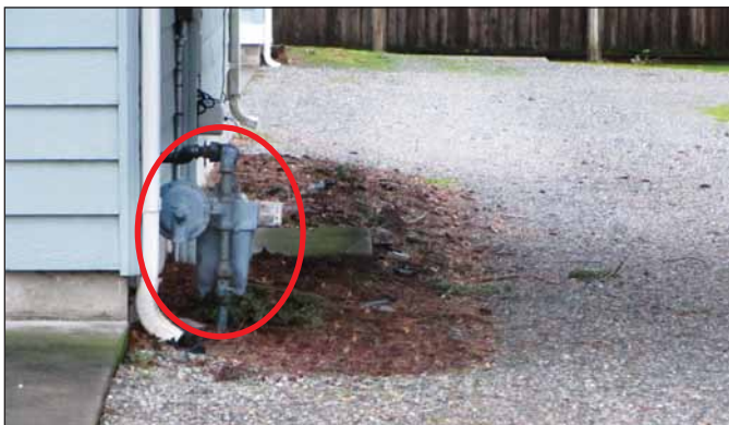
Gas infrastructure vulnerable to outside force damage.
