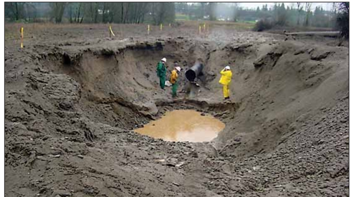
2003 rupture (with no ignition) of a natural gas transmission pipeline near Toledo, WA
