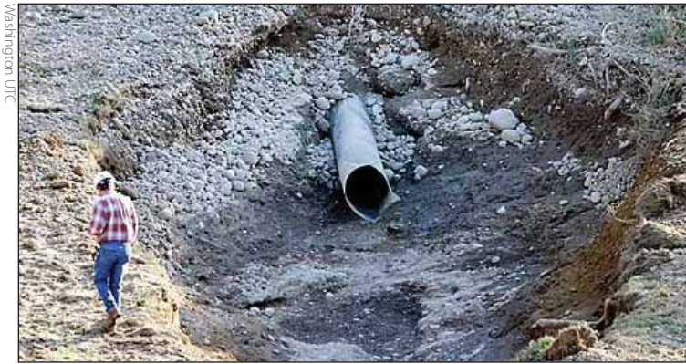
Gas Transmission Pipeline Failure, near Auburn, WA
