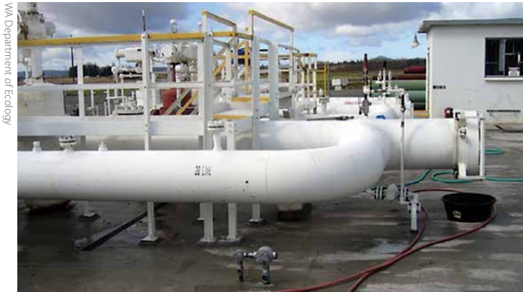
Pig Launchers on a hazardous liquid pipeline near Mt. Vernon, WA
