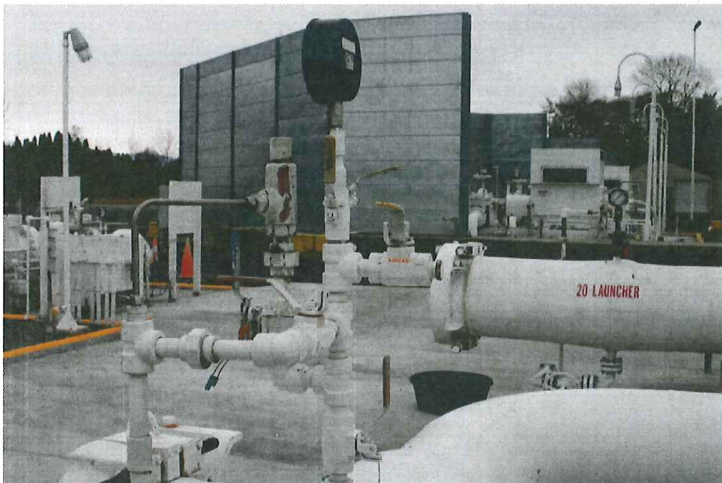
Photo #B-4 of 4 Back ground: 20-inch launcher where the leaks occurred at the sampling port and pressure gauge. The piping has been reconfigured to mitigate vibration from the thermal relief valve. The pressure gauge is isolated from the thermal relief. Foreground: typical "tree" configuration when the failures occurred. Photo taken 4/2/2012 by Al Jones
