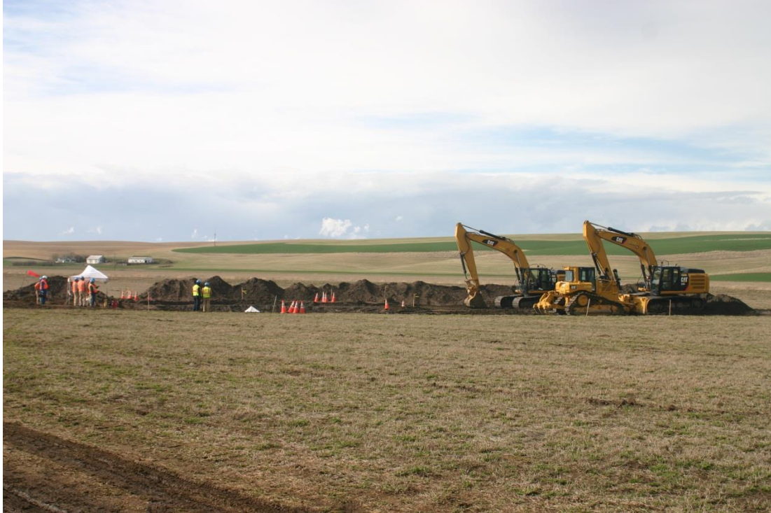
Photo A: Site location of leak on 42-inch Gas Transmission Northwest LLC pipeline, La Crosse, WA Photo taken by Al Jones / UTC, March 20, 2013
