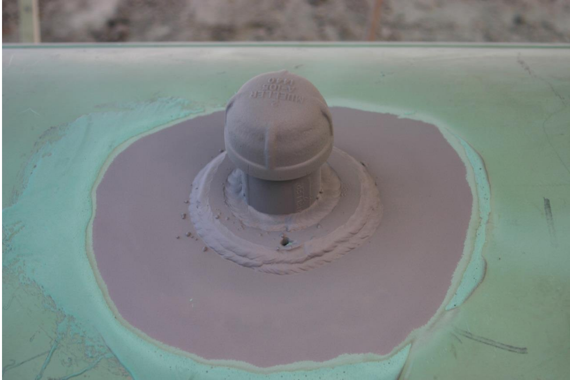
Photo C: 42-inch Gas Transmission Northwest LLC pipeline leak at threaded cap fitting with coating removed.
