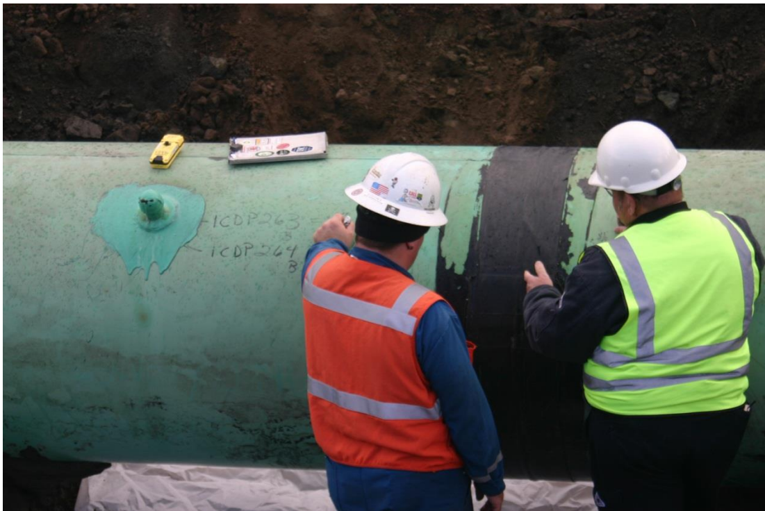
Photo B: 42-inch Gas Transmission Northwest LLC pipeline at threaded cap fitting. Photo taken by Al Jones / UTC, March 20, 2013
