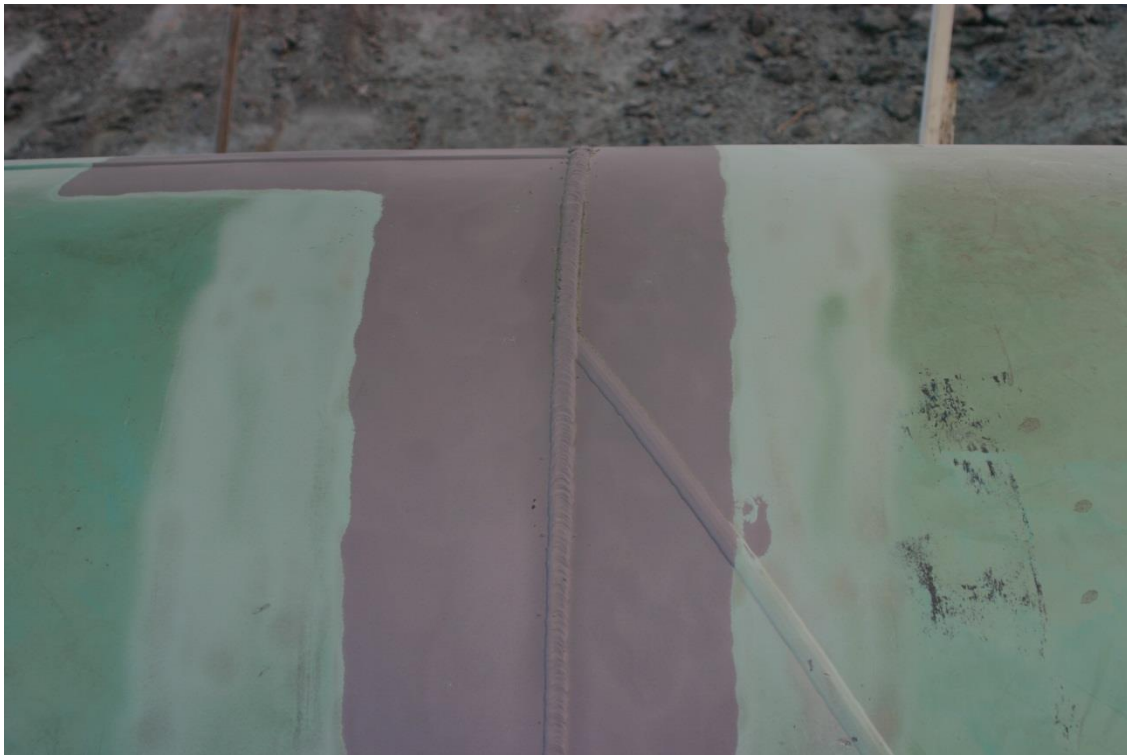
Photo D: 42-inch girth weld and transition between long and spiral seam pipe.
