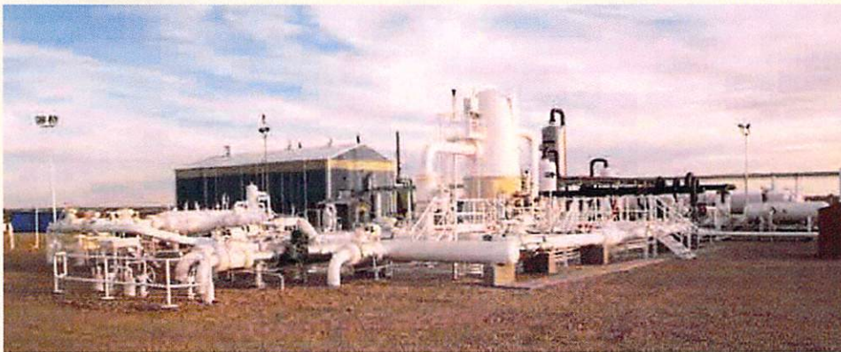
Natural gas compressor station.
