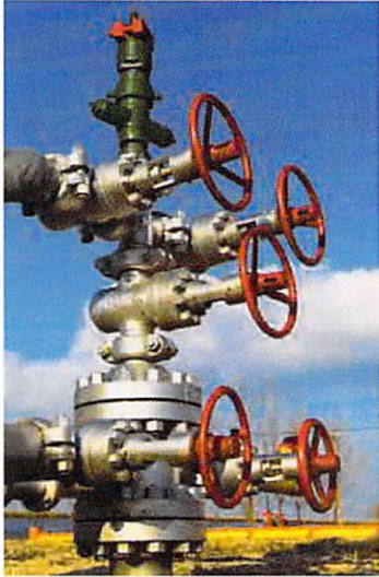
Natural gas wellhead.
