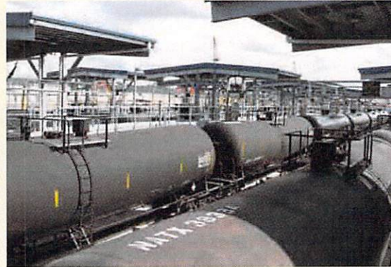
Rail loading facility.
