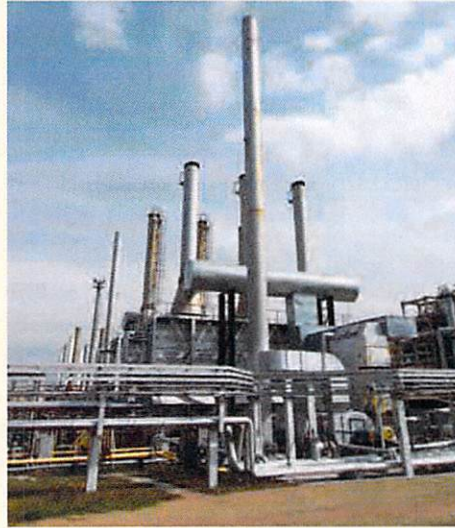
Natural gas processing facility.
